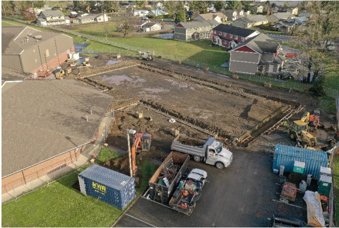
These drone aerial photos were taken on November 19 and they show 75% of the concrete footings poured with more forming underway.
