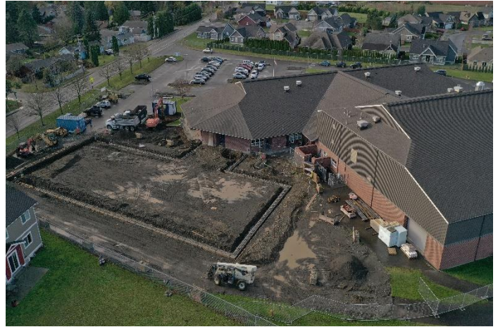
Another view showing where the Everson 10 classroom addition is located in relation to the school and where the hallway will connect.
