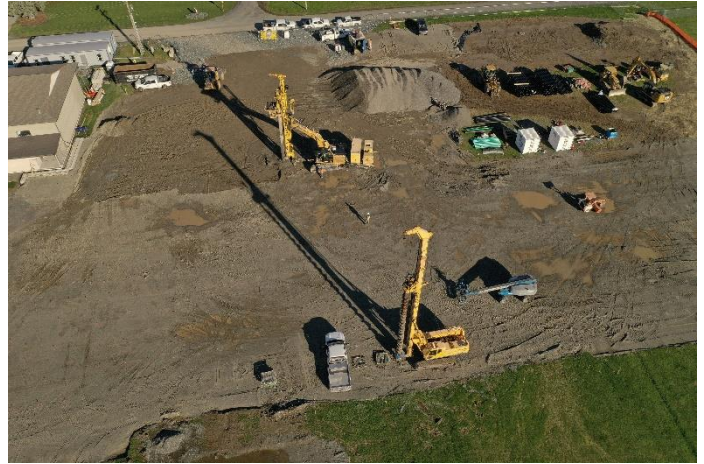
The pre-drill rig is at the forefront and the aggregate pier rig is at the back.
