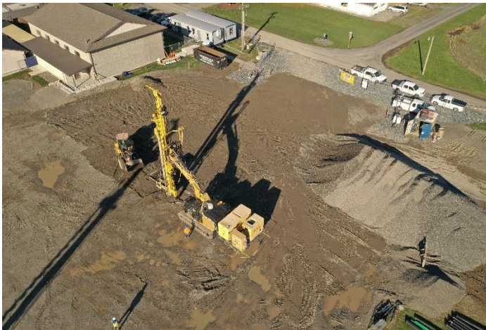
A close up of the aggregate pier rig in action with the loader in front.
