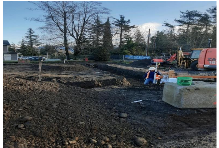
The southwest corner forms started going in today and will complete the perimeter footings and will be poured soon.
