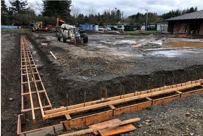
Form work on the majority of the classroom addition was completed on November 18 and was inspected and approved.
