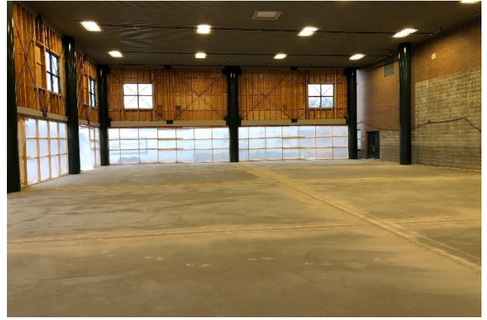
The new level concrete gym floor is finished and now has the saw cut expansion joints completed.
