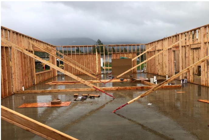
The exterior wall framing is looking good and interior wall framing is underway in the classroom addition.
