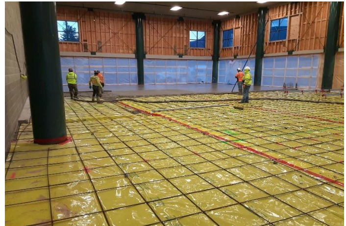
The vapor barrier and rebar installation and inspection was completed this week. Concrete placement was done utilizing a concrete pump.
