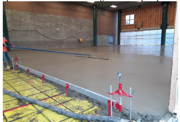
The next step after concrete is placed is utilizing the concrete float.
