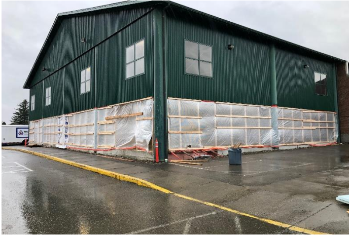
Tiger Construction weatherized the covered play area to allow for a concrete pour despite the rain and wind this week.
