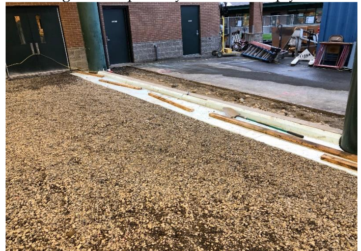
Perimeter insulation has been installed as part of the preparation for the new gym concrete slab.
