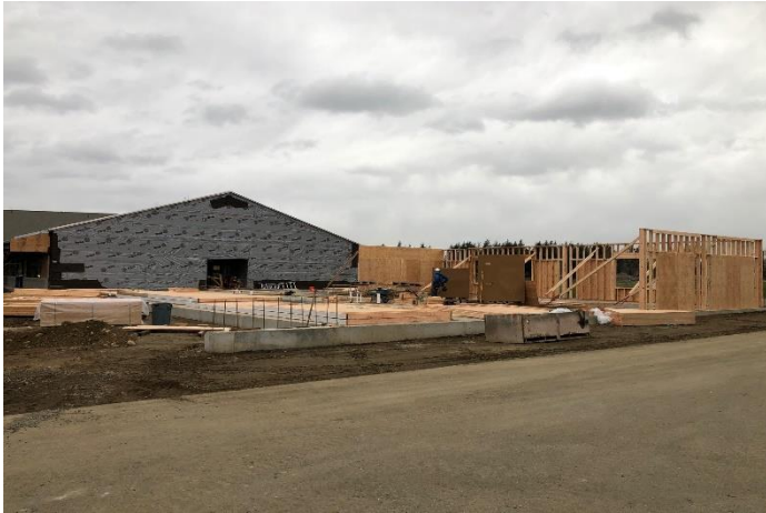
Wall framing has begun and the first walls went up today with many more built and ready.
