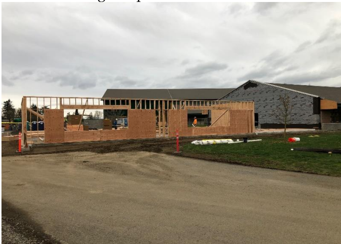
Another view of the east wall with the large window openings for each classroom.
