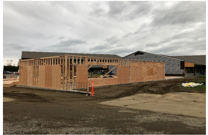
Portions of the south and east walls are now standing and are partially sheeted with plywood.
