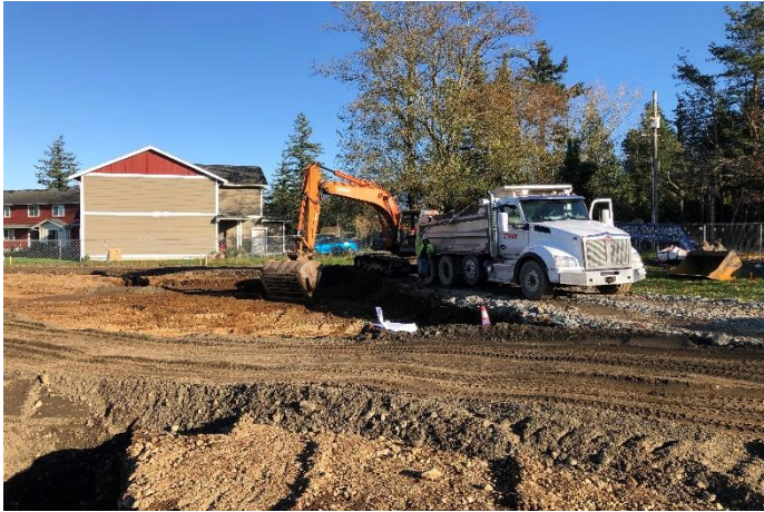
Over excavation is taking place at the South East corner of the new 10 classroom addition.
