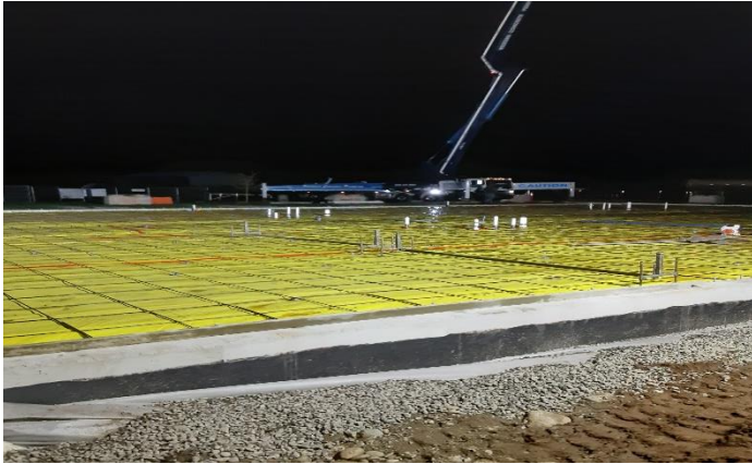
6:00 a.m.: Vapor barrier complete, rebar in place, inspections done and ready to pour.
