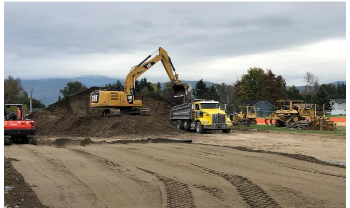
Load out and removal of the soft soils was underway this week.
