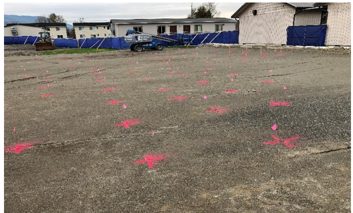
Layout work is complete on the compacted building pad and is ready for aggregate pier installation to start next week.
