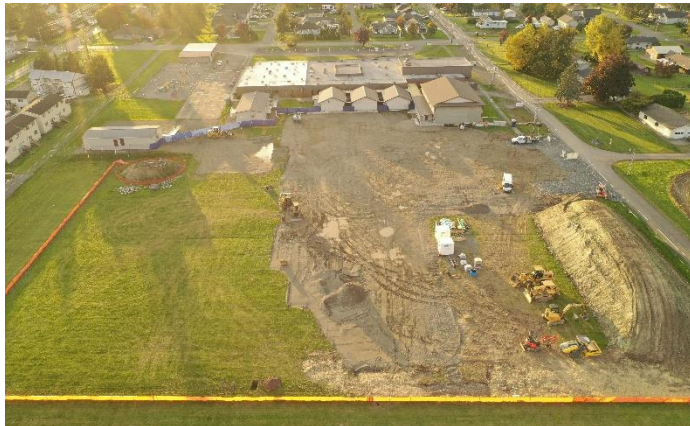
This aerial view shows the initial site preparation under way that included excavating 2 feet of sod and soft soils at the building pad & replacing with compacted gravel.
