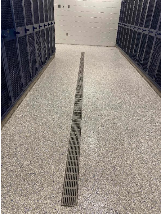
SFHS – Lockers installed in area A locker rooms
