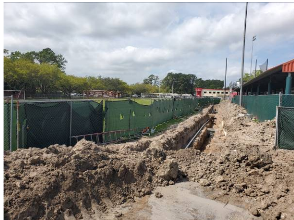
Utilities to the Tennis Field House from Baseball
