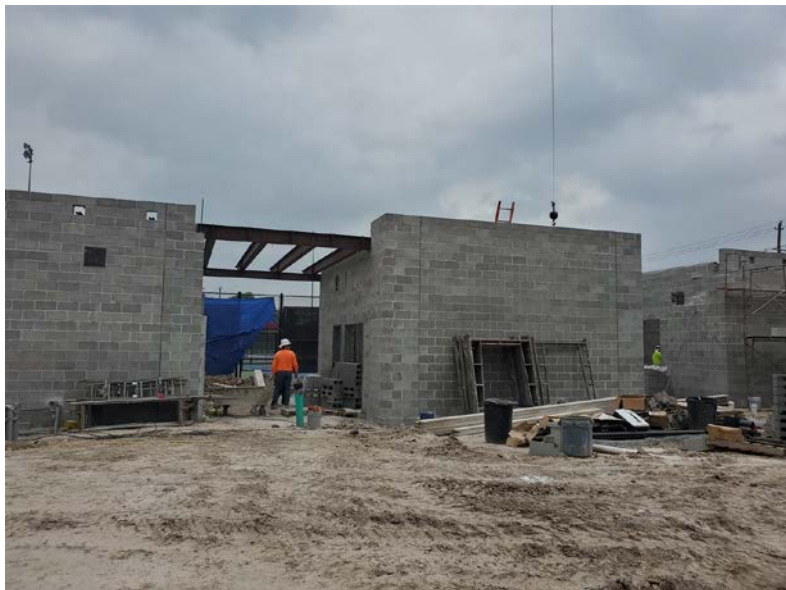
New tennis field house
