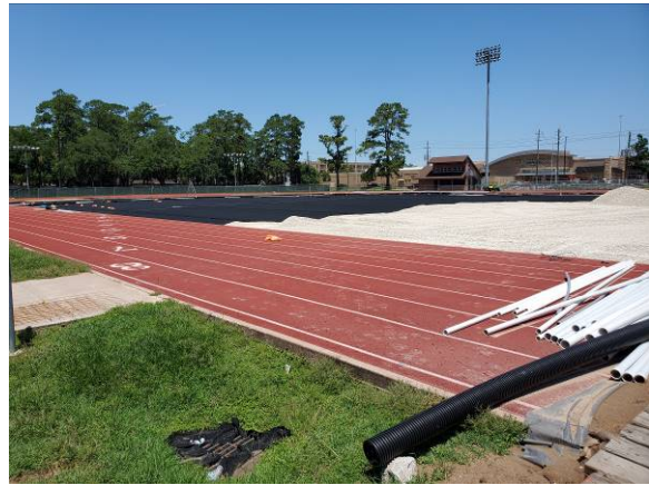
Turf field drainage fabric and rock
