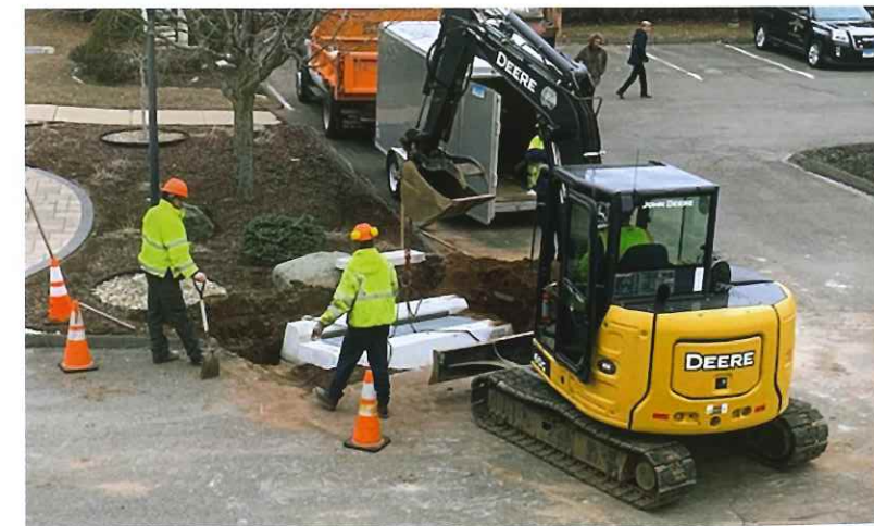
A catch basin is repaired as part ongoing efforts to ensure effective road drainage throughout Ellington.
