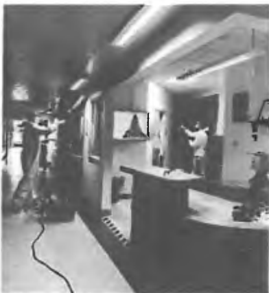
Initial treatment of the ward with the organosilane compound using the electrostatic sprayers.
