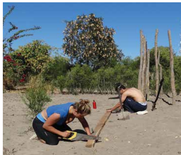
Preparing the rafters for a house for the homeless in Mwandji, Zambia.
