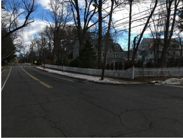
Fern Street Sidewalk Gap Elimination South Sidewalk Installation between Hamilton Avenue and Walbridge Road
