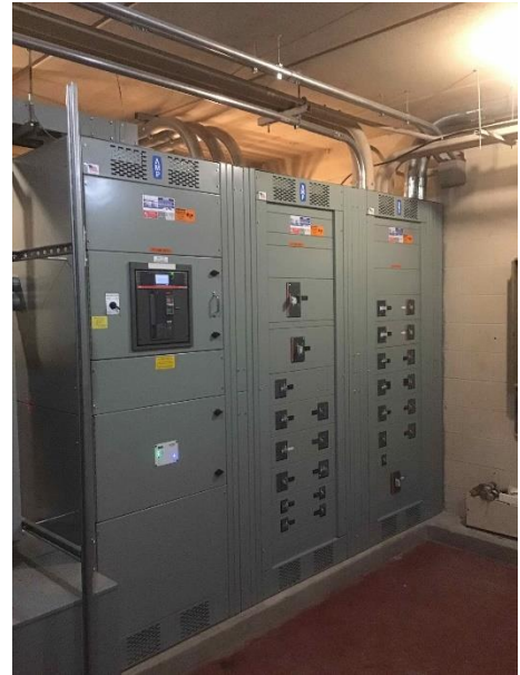
SFHS Electrical Panel
