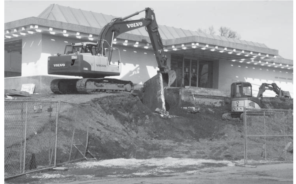
The reconstruction began with the demolition of the steep uphill which led to the old entrance.
