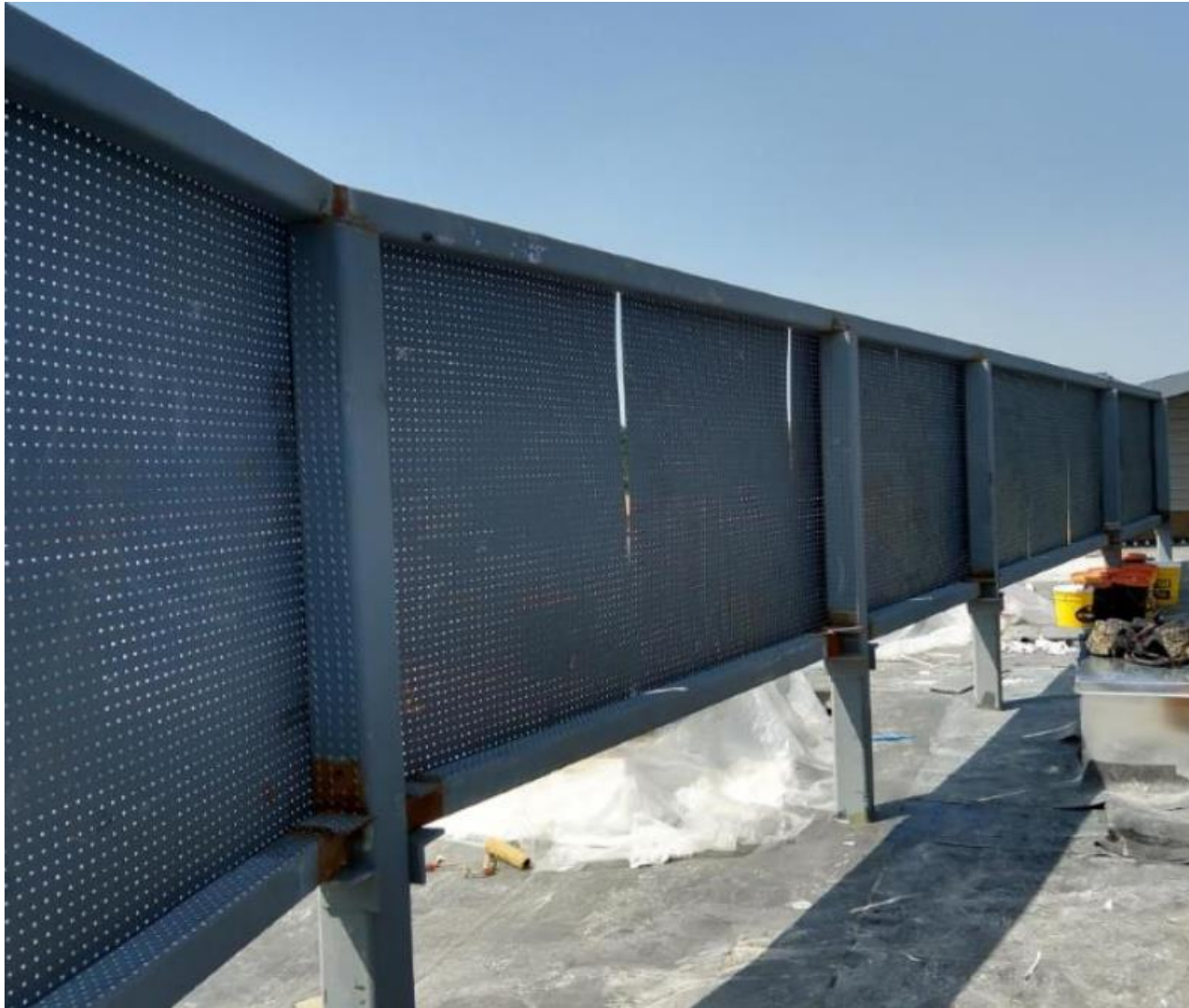
Mechanical screens on roof.
