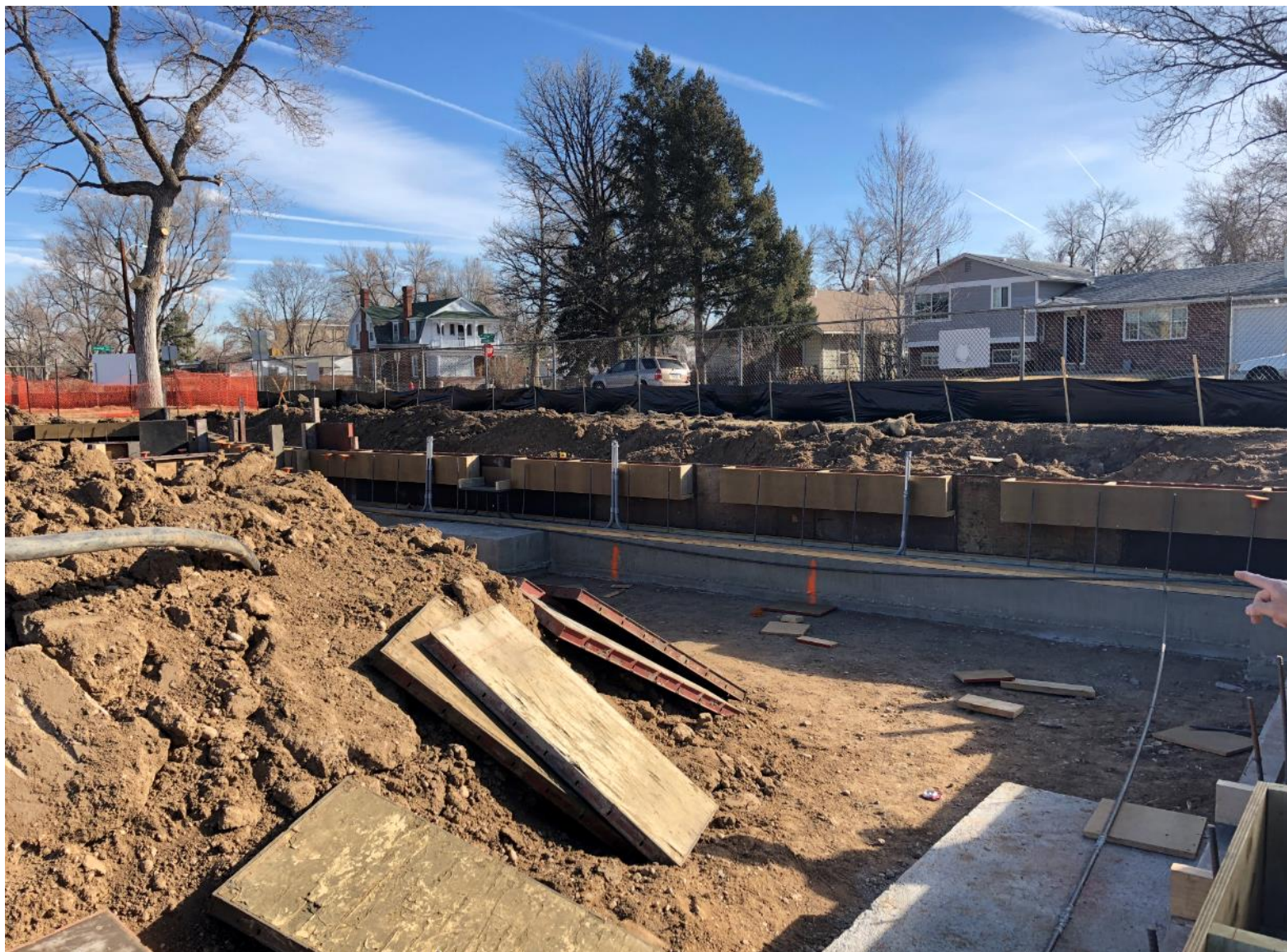
Conduit stub-ups at East wall.
