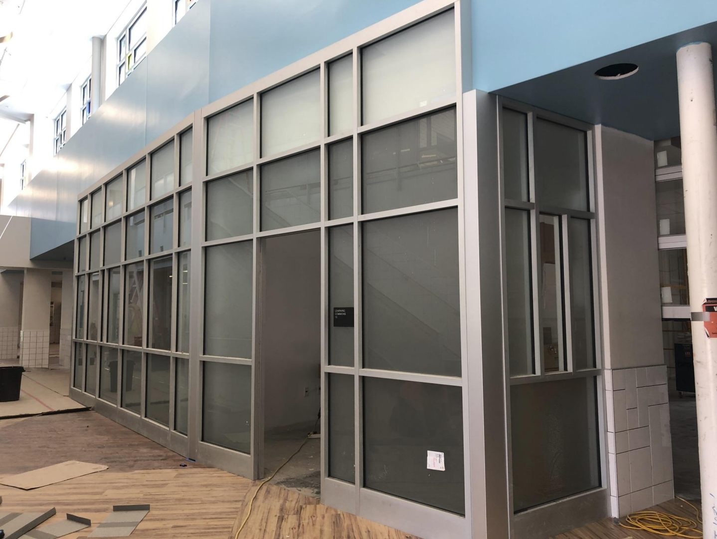
Grand Hall – Storefront glass system, paint, room signage, and flooring fully installed.
