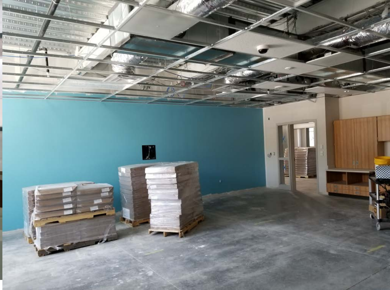
South Classroom Wing (L1) – Classroom; Flooring to be installed soon. Painting and cabinets complete.
