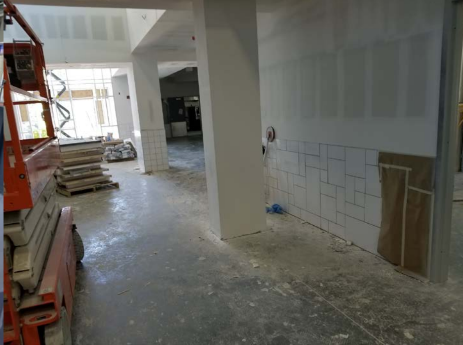
Grand Hall – North Facing View; Tile being installed and painting to begin soon.
