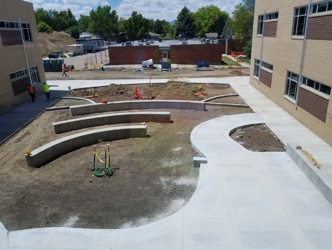
West Elevation – Plaza Between Classroom Wings; Sitework continues, concrete paths newly poured.
