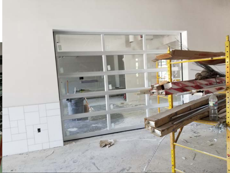
STEM Classroom – Garage doors and tile newly installed.
