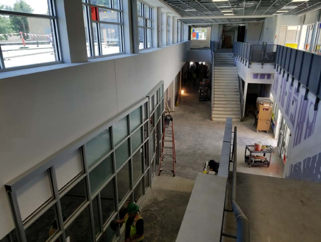
Grand Hall – South Facing View; Storefront glass and frames on lower level and ceiling being installed and painting in progress.
