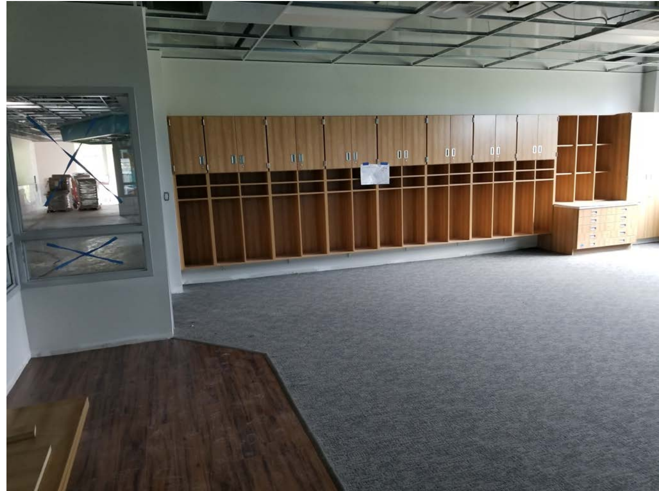
North Classroom Wing (upper level) – Classroom; Ceiling tile to be installed soon.
