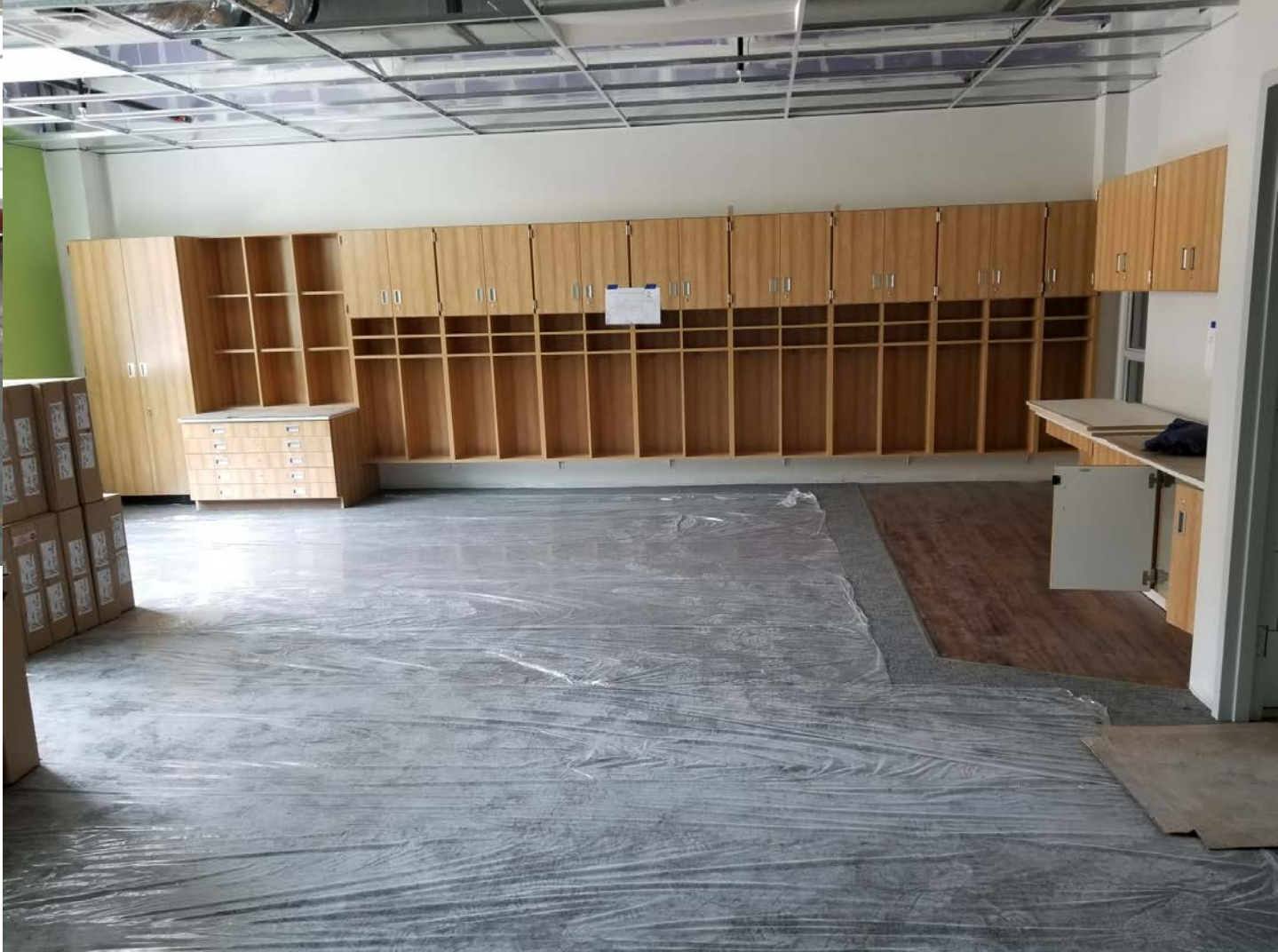
North Classroom Wing (lower level) – Classroom; Ceiling tile to be installed soon.
