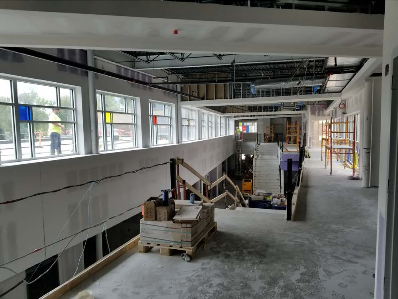
Grand Hall – South Facing View; Drywall recently completed, painting to begin soon.
