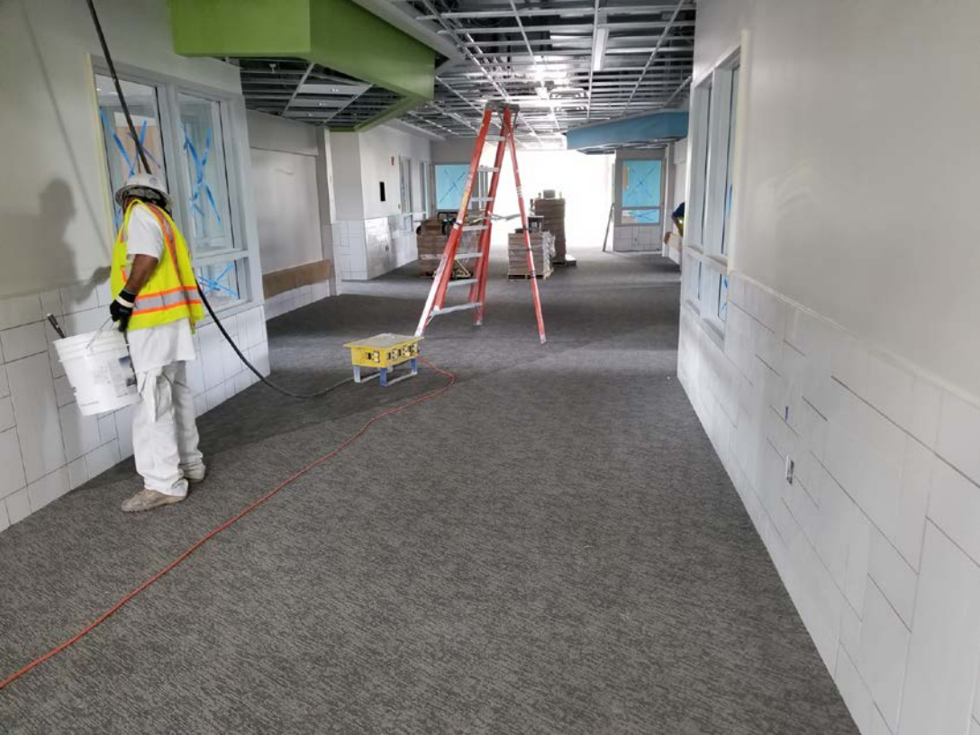
North Classroom Wing (upper level) – Painting finishing, ceiling tile to be installed soon.
