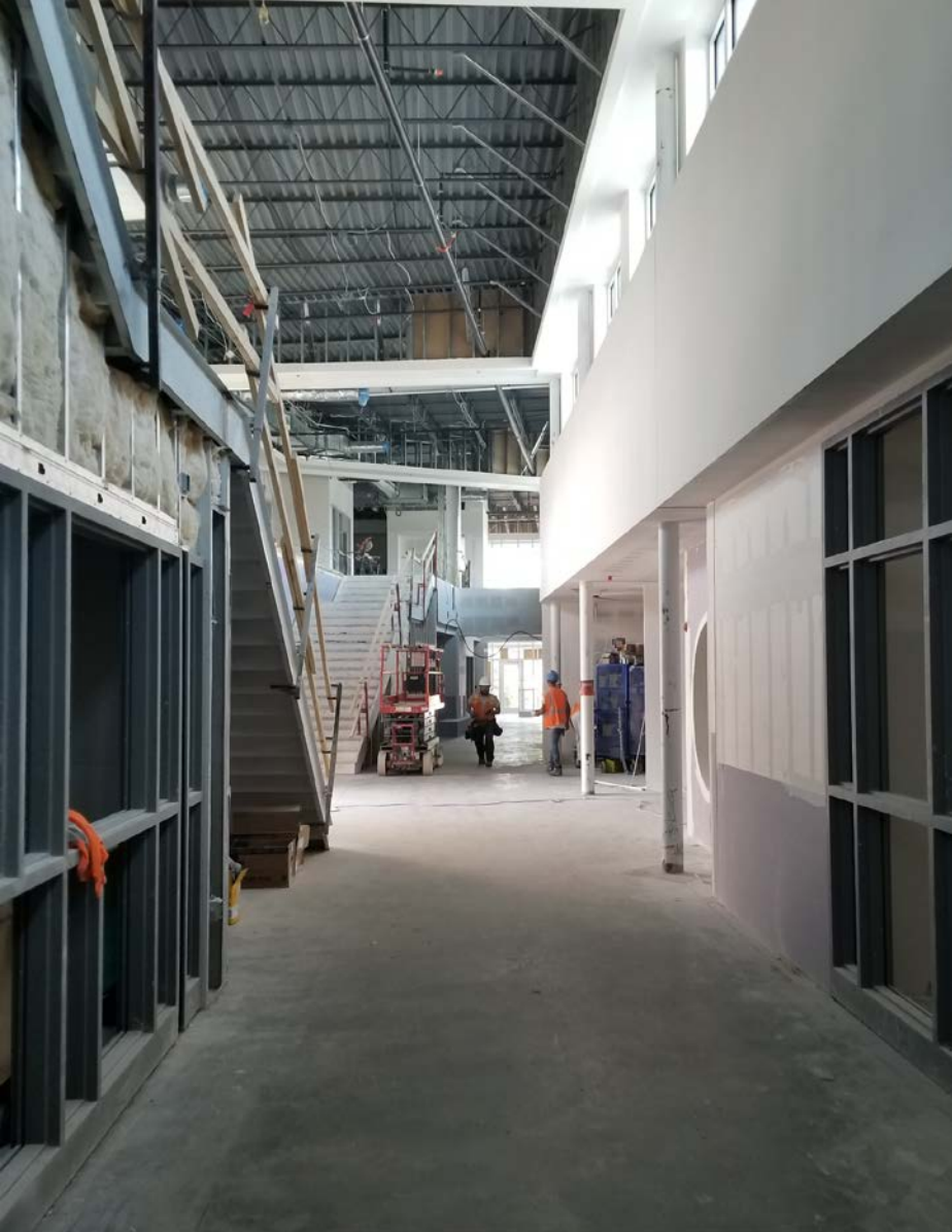
Grand Hall – South Facing View; Drywall install finishing, ceiling being installed, and painting to begin soon.
