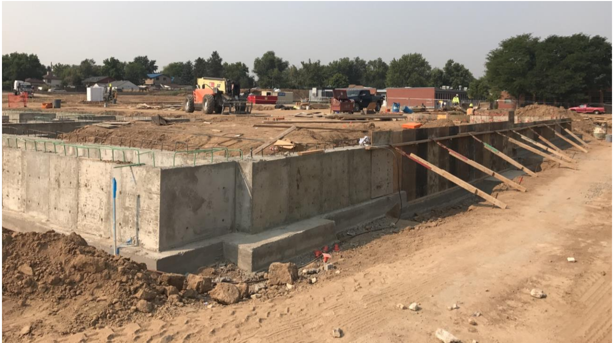
Walls being formed to continue around NE Corner to North to NW Corner
