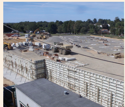
Work is progressing as the foundation and walls for the new Lynnewood Elementary School are put in place.
