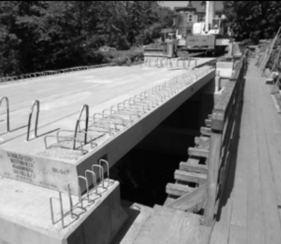
Work on the Boston Neck Bridge is nearing completion. It is expected to be finished early in the next fiscal year.
