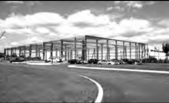
The steel frame of the Windsor Marketing Group will add 88,000 square feet to the company's existing building on South Street.
