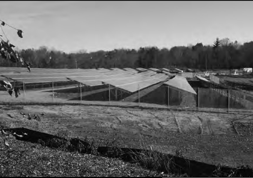
Pictured above is a portion of the solar farm being built by Lodestar west of North Street and south of Halladay Avenue West.
