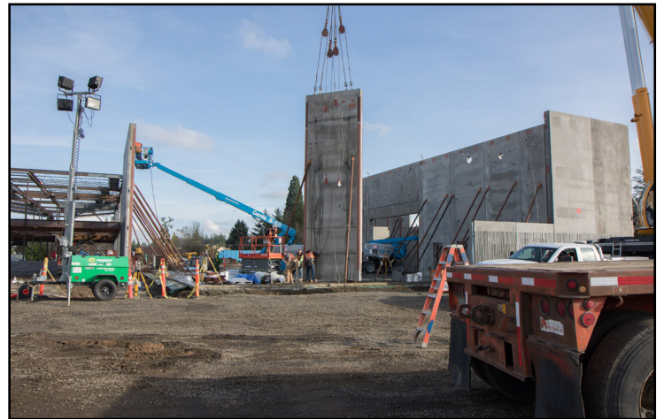
Precast panel in gym
