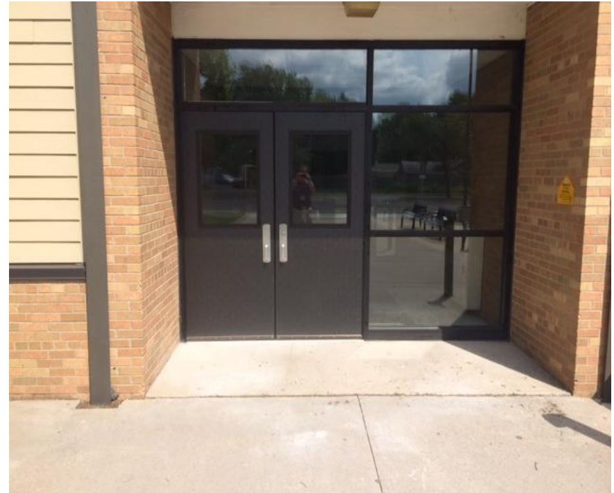
Sunrise Park Middle School Exterior Doors
