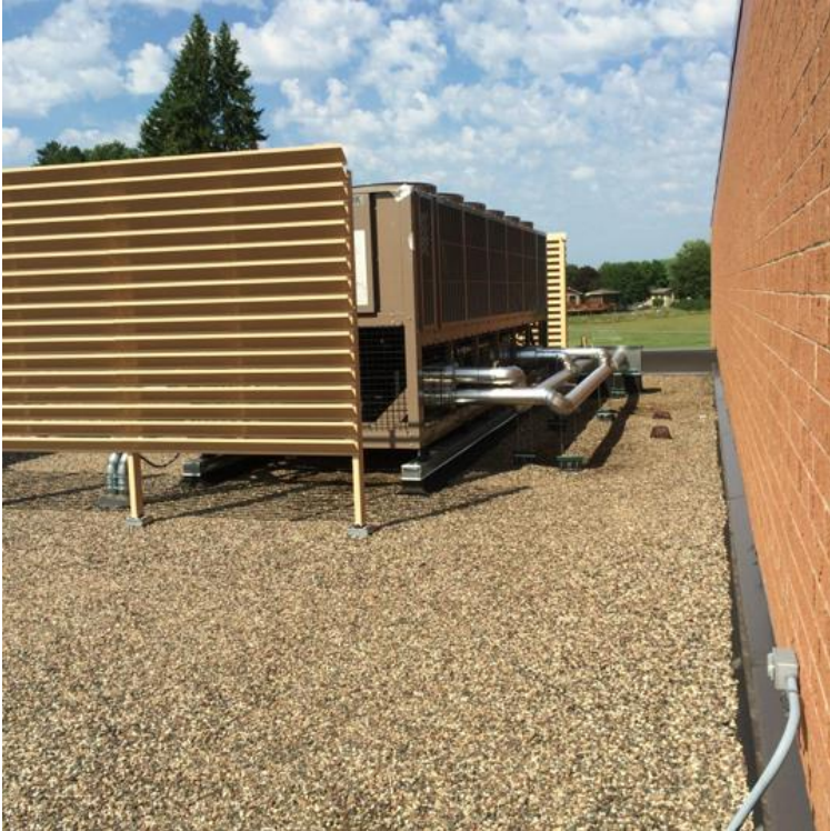
Otter Lake Elementary HVAC
