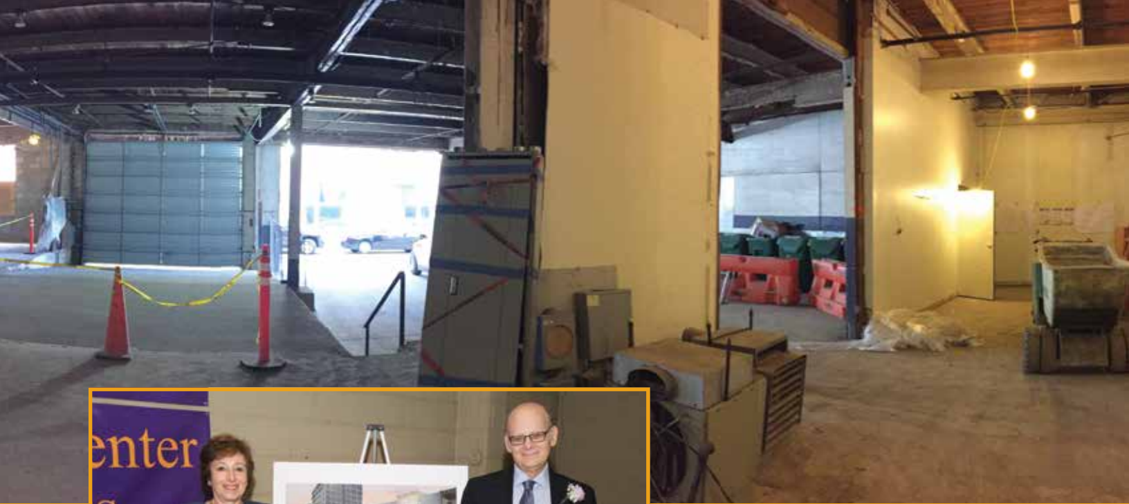
Pictured above is the ground floor of The Howard Center for the Arts that will serve as a parking facility.
