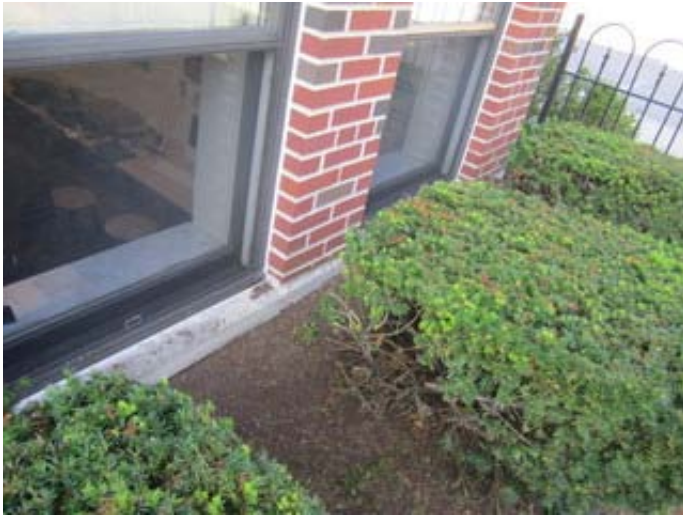
Foundation at Ground Floor Showing No Signs of Repair
