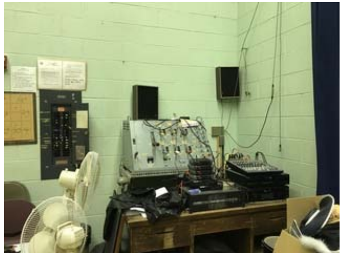
Stage Lighting Control Panel And Breakers
