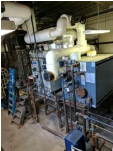
Existing Steam Boilers in the Mechanical Room at Smith Elementary School
