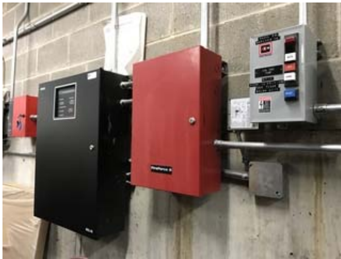
Main Fire Alarm Panel
