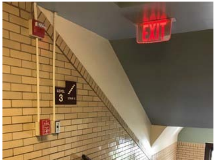
Typical Manual Pull Station, Horn And Strobe Devices
