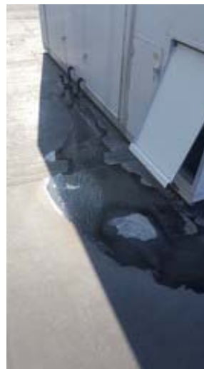
Standing Water on Roof Over the 2003 Addition
