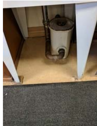
Solids Interceptor Under the Sink in the Art Room
