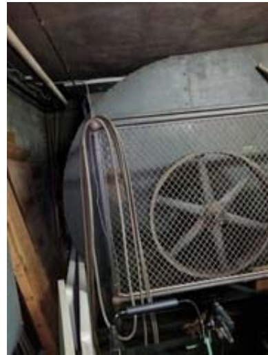
Fan Providing Central Air to the Original Building at Smith Elementary
