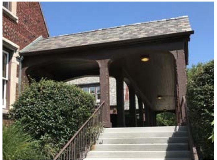
Pedestrian Walkway Lighting
