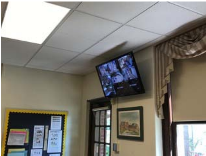
CCTV Monitoring System In Administrative Area
