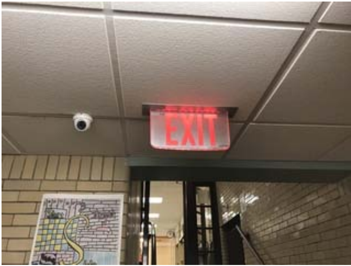
Typical Exit Sign
