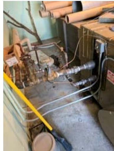
Existing Heating and Ventilating Unit Located in the Mechanical Room Behind the Music Classroom
