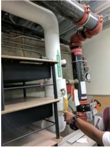
Domestic Water Service and Fire Service Entrance at Smith Elementary
