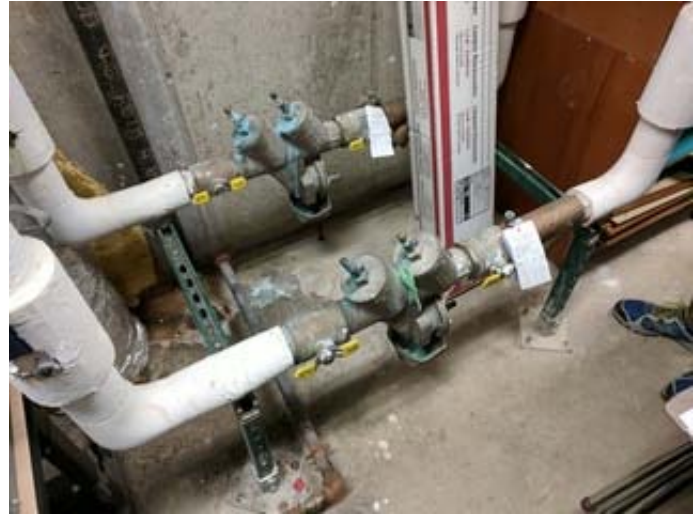
Domestic Water Backflow Preventers at Smith Elementary
