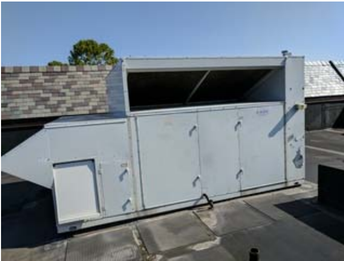
Aeon Rooftop Unit Serves the 2003 Building Addition
