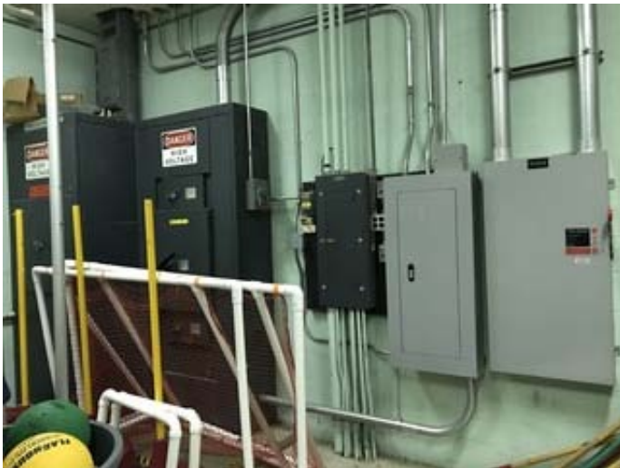
The Building's Electrical System
