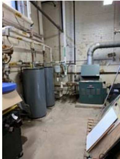
Existing Hot Water Heater and Storage Tanks in the Mechanical Room at Smith Elementary School
