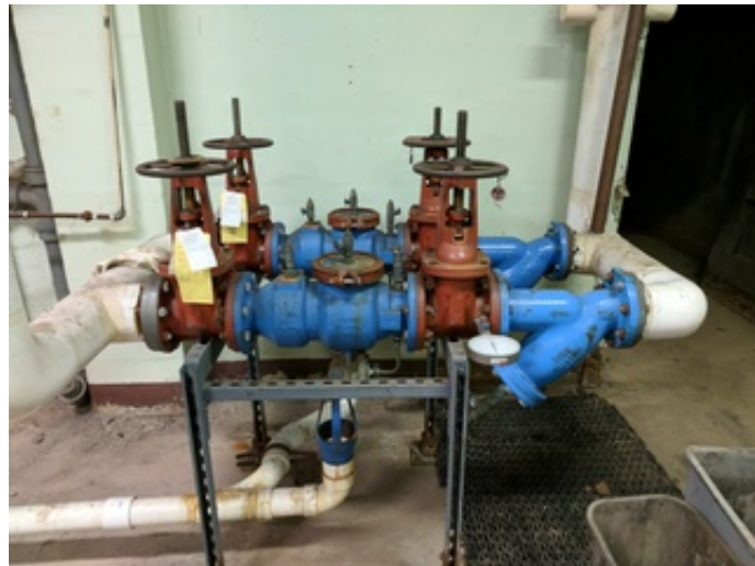
Dual 4" Backflow Preventer Located in the 2003 Building Addition Mechanical Room
