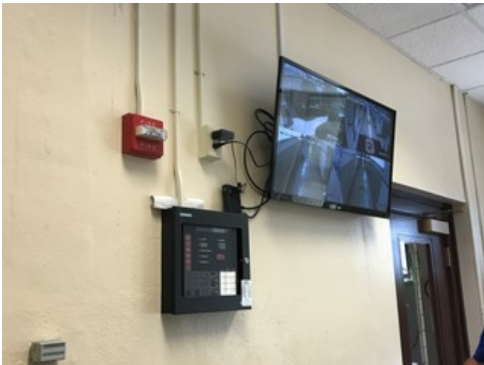
CCTV Monitoring System In Admin Office
