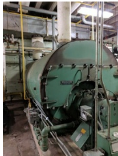
Kewanee Steam Boiler in the Original Construction
