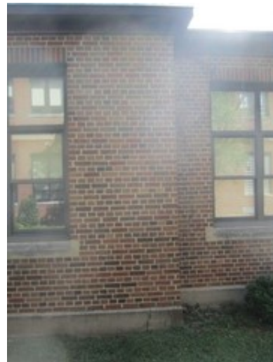
Foundation Crack, Courtyard Side of 1932 Addition
