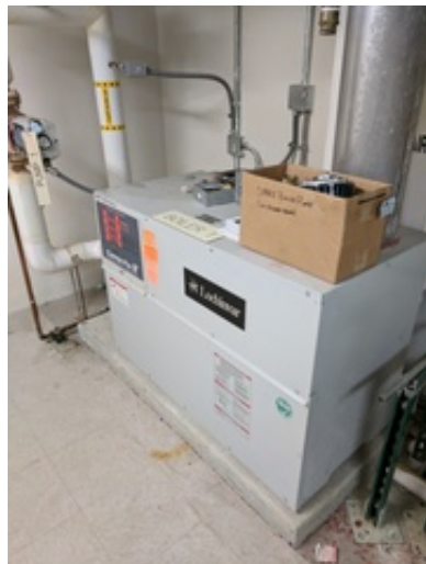
Lochinvar Hot Water Boiler in the 2003 Building Addition
