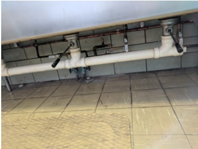
Sanitary Drain Piping Below the Three Compartment Sink
