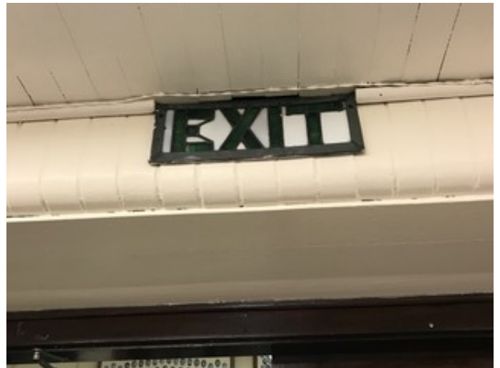
Typical Green Lettered Exit Sign
