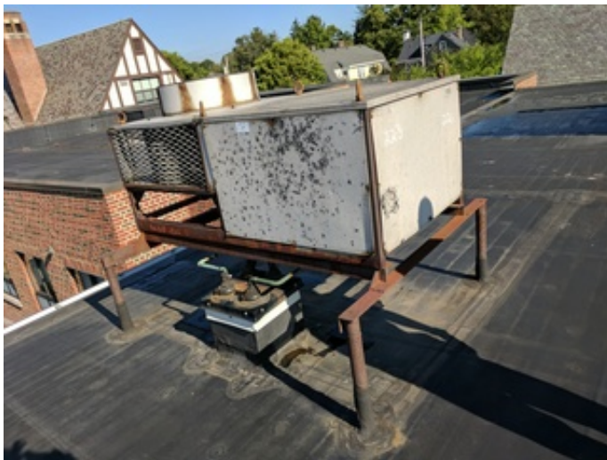
Air Cooled Condensers Serving the 1969 Building Addition
