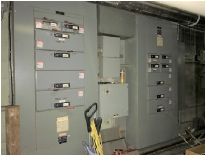
Electrical System To The 1960 Addition
