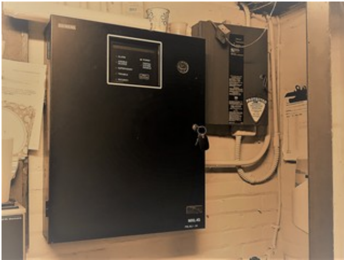
Fire Alarm Control Panel
