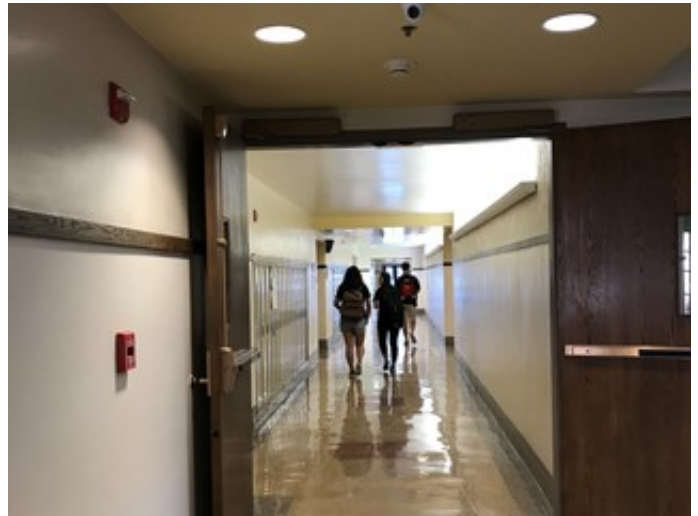
Typical Fire Alarm Devices
