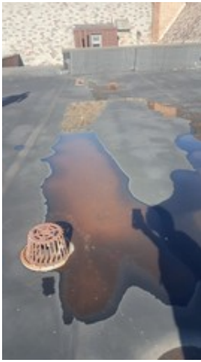
Ponding on Roof Over the 2003 Addition
