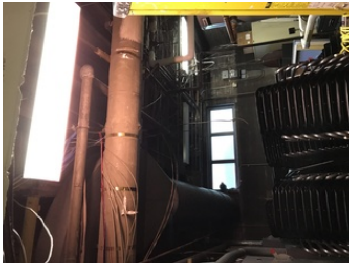
Pipe Fittings in Basement
