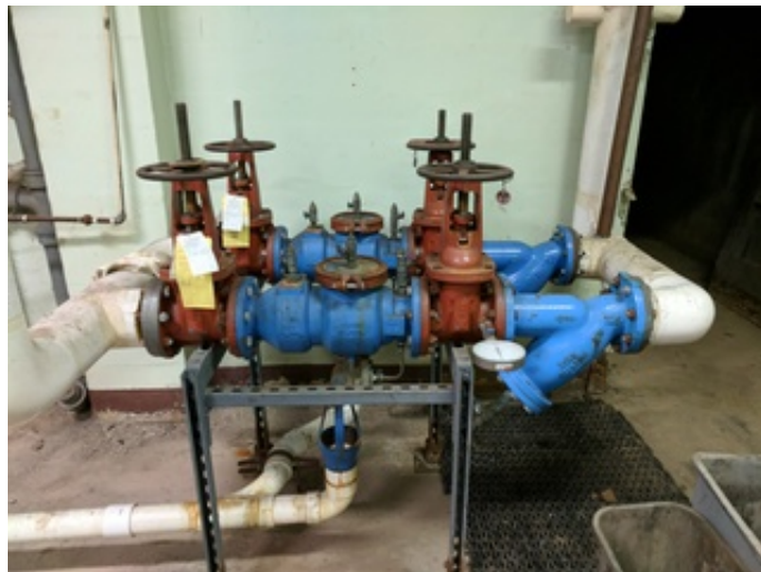
Backflow Preventers at Oakwood HS/JHS
