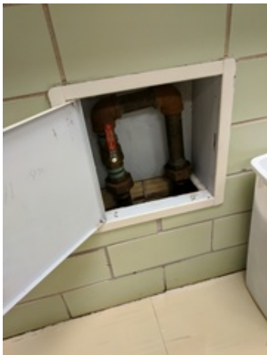
Master Shutoff For Gas in A Science Laboratory
