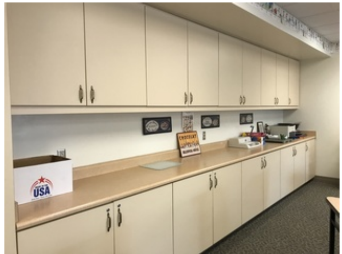
Typical Classroom Receptacles
