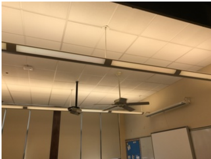
Typical Classroom Lighting
