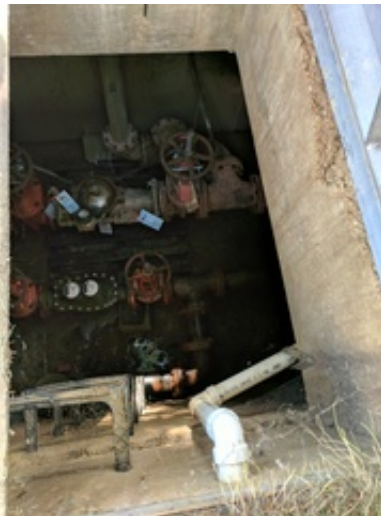
Water Meter and Fire Service Connection Pit (Outside)
