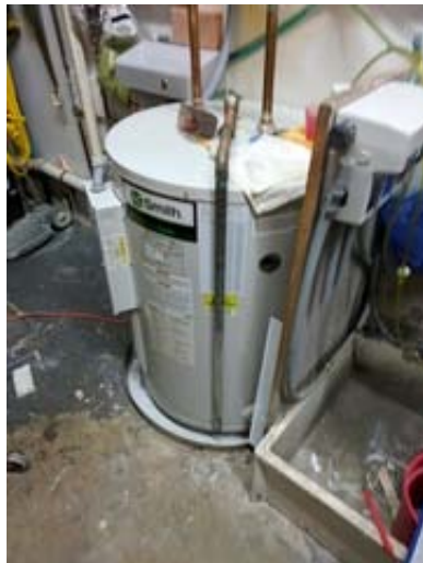
Electric Water Heater In the Janitor Closet
