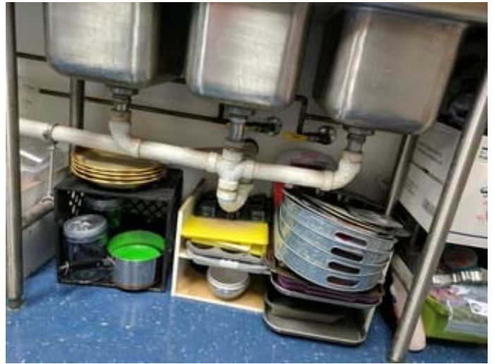
PVC Drain Piping
