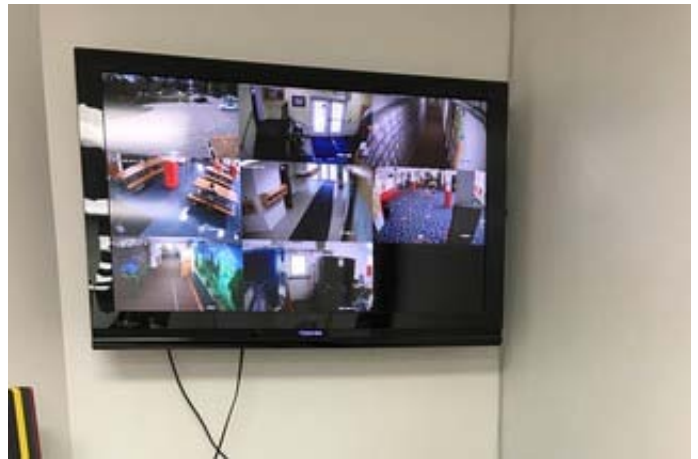
Security Monitor At Reception Area
