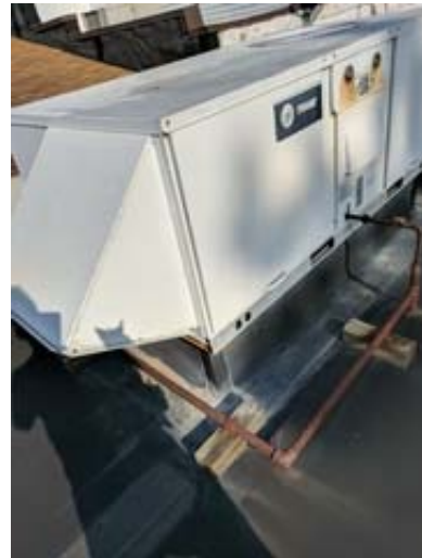
Gas Piping to Trane Rooftop Unit
