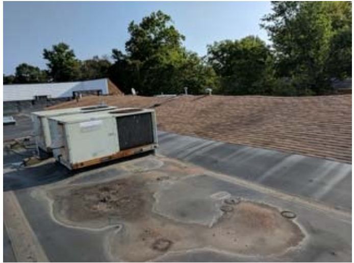
Two Bryant Rooftop Units at Lange School
