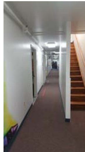
Non-compliant Stair and Corridor
