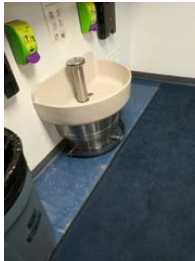
Typical Wash Fountain at Lange School
