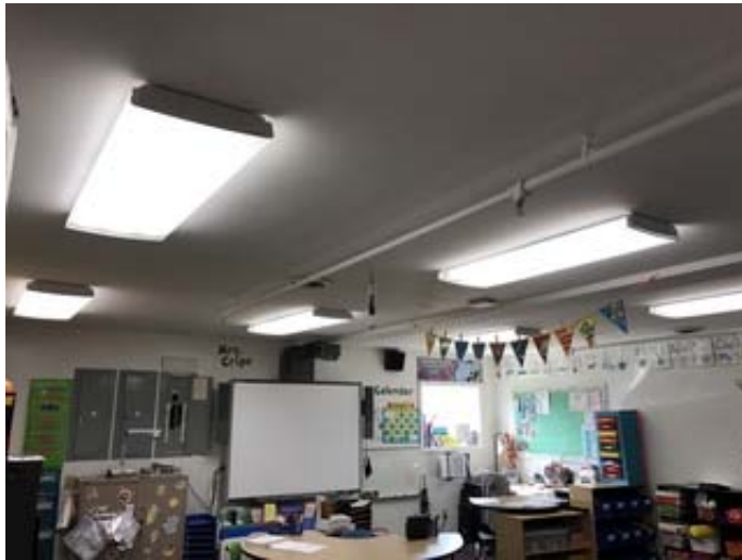
Typical Ceiling Devices And Smartboard
