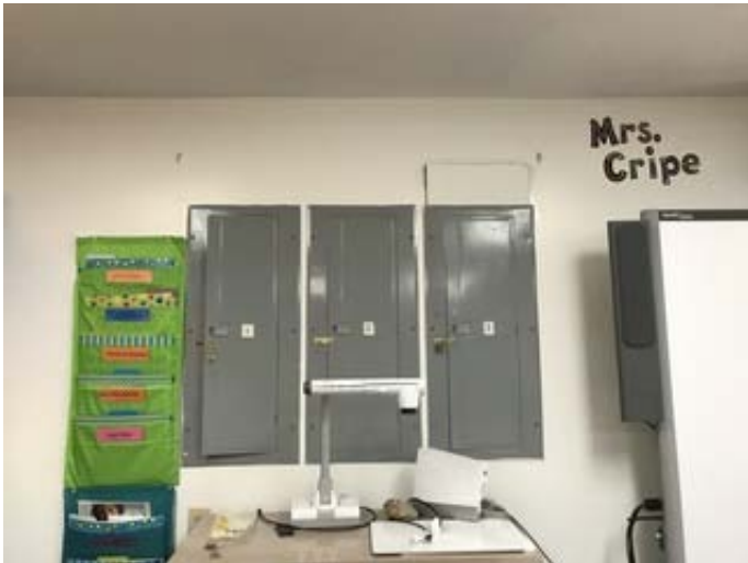
Building's Electrical Panels
