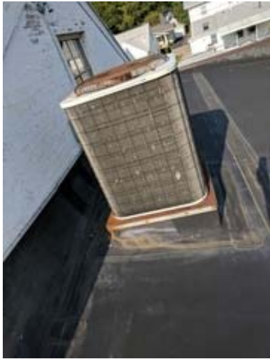
Air Cooled Condensing Unit on Roof Serves Air Handling Unit in the Mezzanine
