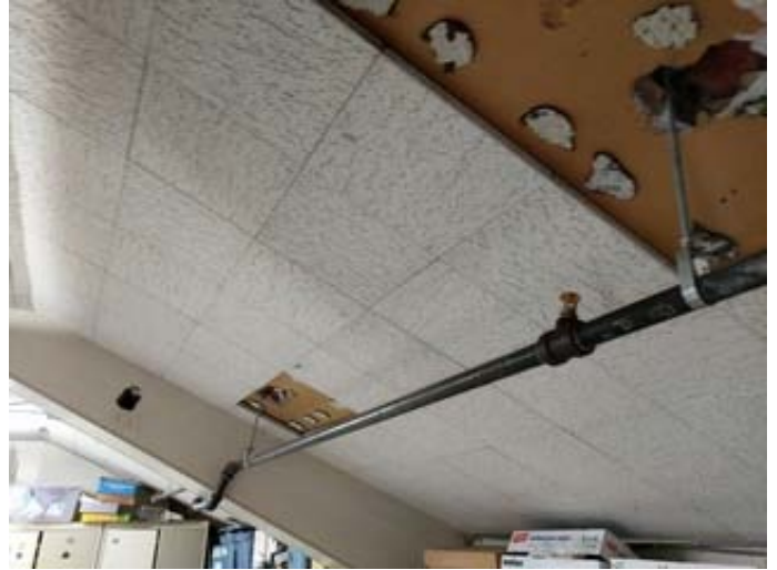
Sprinkler Piping in the Mezzanine at Lange
