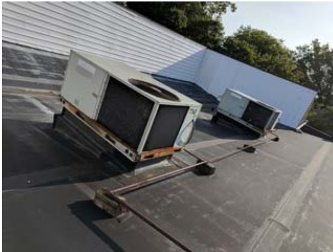
Gas Piping to Bryant Rooftop Units
