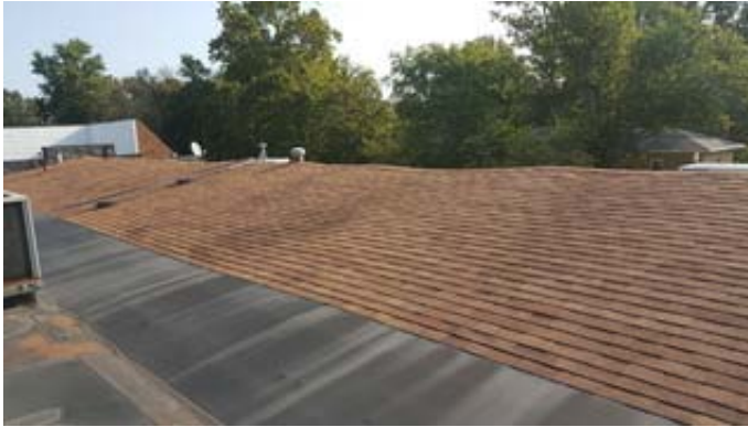
Sagging Roof Framing
