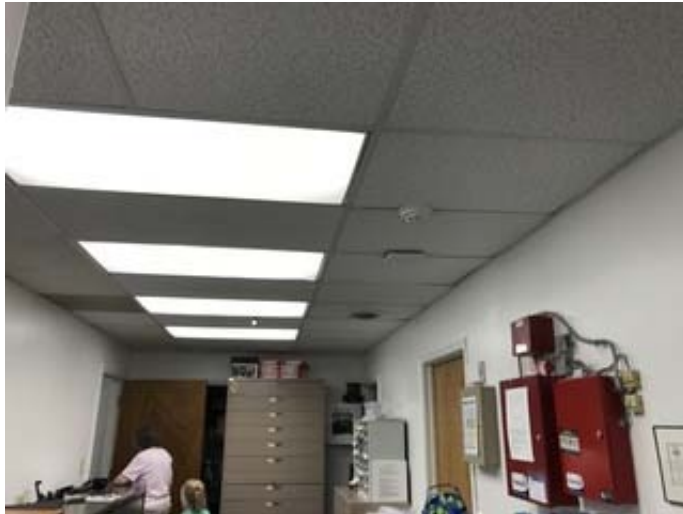
Fire Alarm Panel And Smoke Detector
