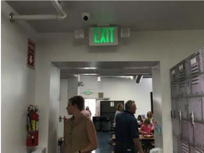
Typical Exit Sign
