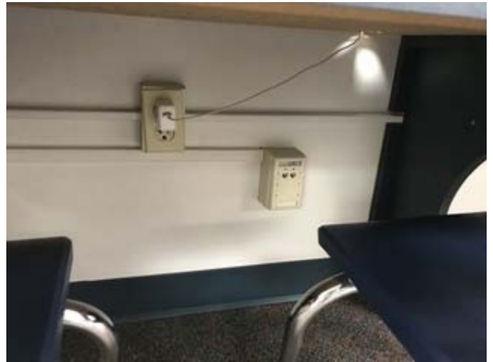
Typical Classroom Data Ports
