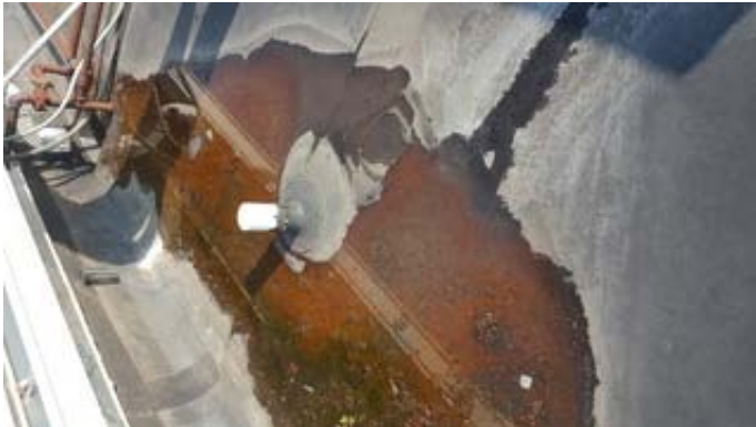
Area of Ponding
