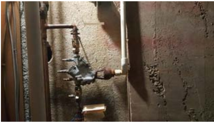
Backflow Preventer at Lange
