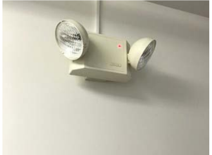
Typical Emergency Lighting
