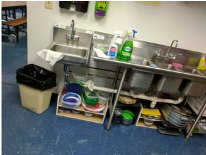
PVC Drain Piping
