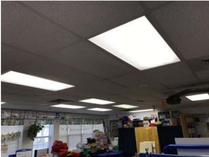
Typical Classroom Lighting
