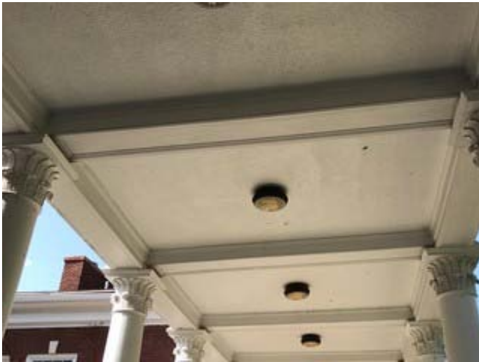
Lighting At Pedestrian Walkway
