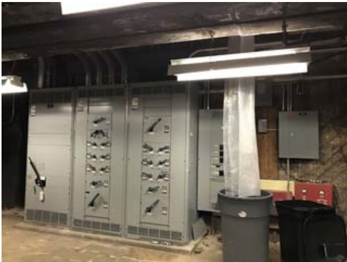
Main Electrical System
