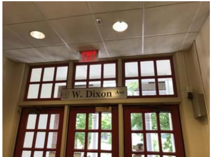
Typical Emergency And Egress Lighting In 2003 Addition
