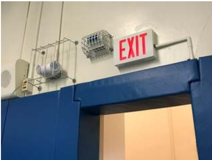
Typical Emergency And Egress Lighting In Original Construction
