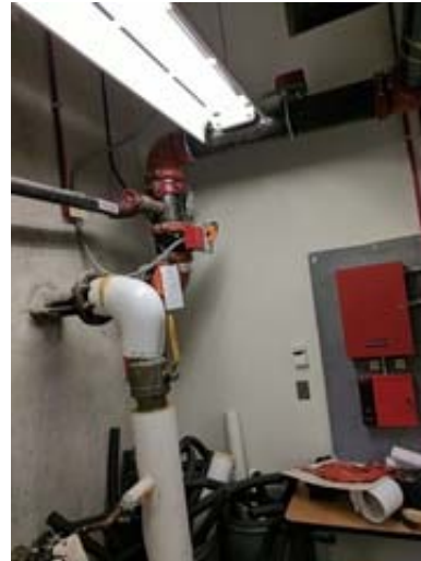
Location Where the 4" Domestic Water and 6" Fire Service Pipes Enter the Building
