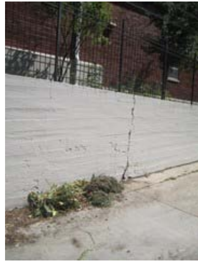
Cracked Retaining Wall
