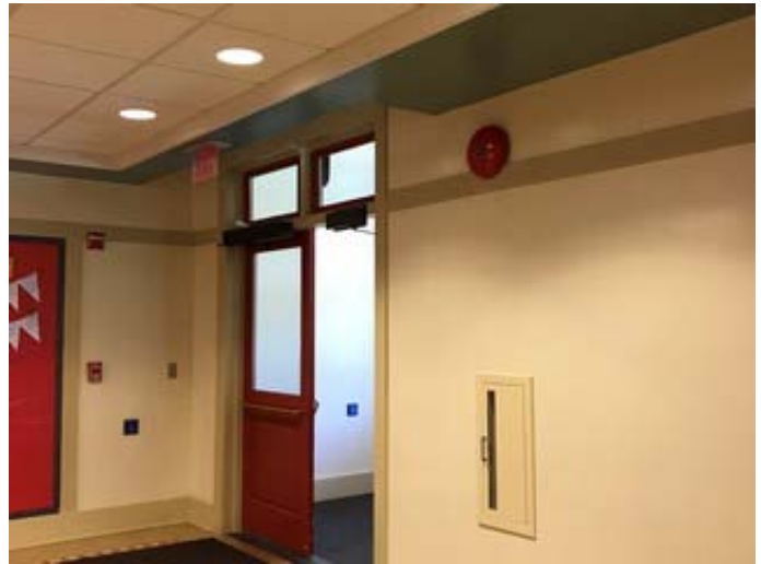
Typical Fire Alarm Devices
