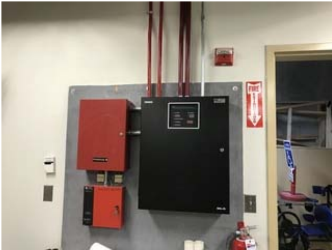
Fire Alarm System
