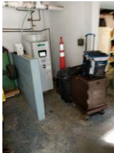
80 Gallon Electric Water Heater in Storage Room below the Kitchen at Harman Elementary School
