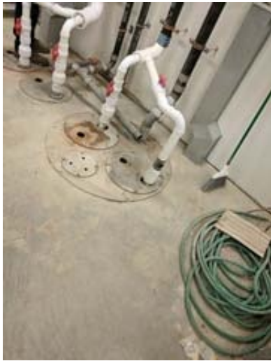
Sewage Ejector Pumps at Harman Elementary
