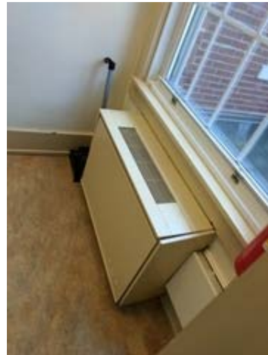
Unit Ventilator At Harman Elementary
