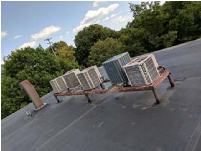
Air Cooled Condensing Units Serving rooms 34, 35, the Computer Lab and South Library
