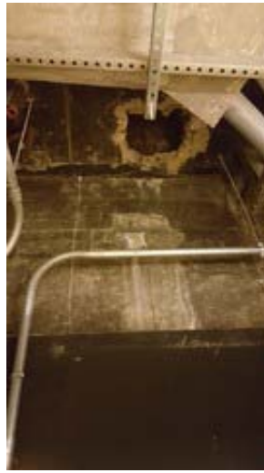
Pipe Fittings in Basement
