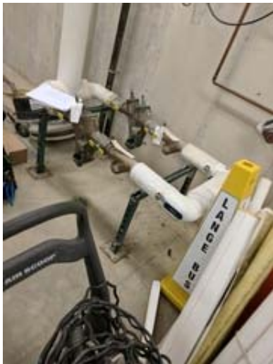
Backflow Preventers at the Domestic Water Service Entrance
