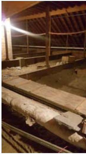
Pipe Fittings and Insulation in the Attic
