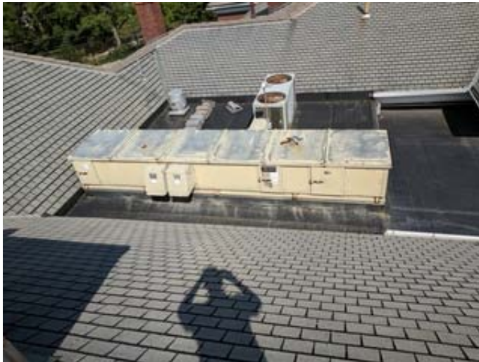
Rooftop Unit Serving the 1998 Building Addition
