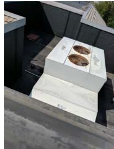
Aaon Rooftop Unit Serves the 2003 Building Addition
