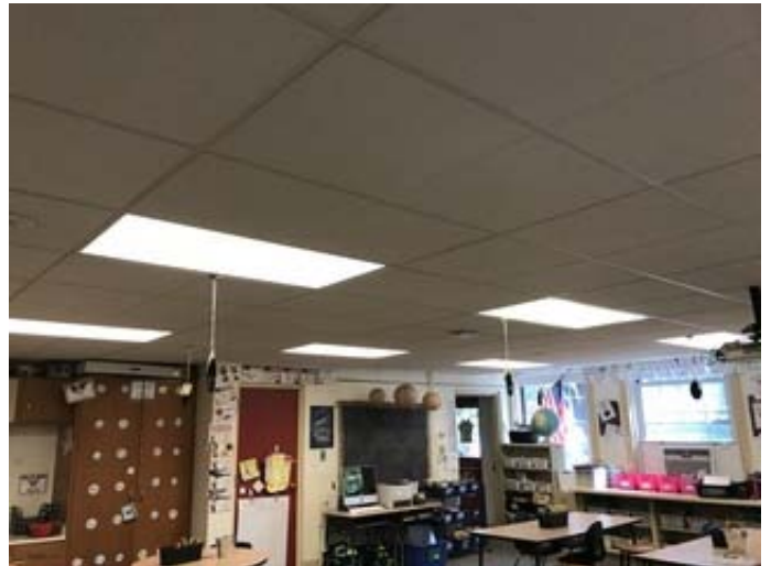
Typical Classroom Lighting
