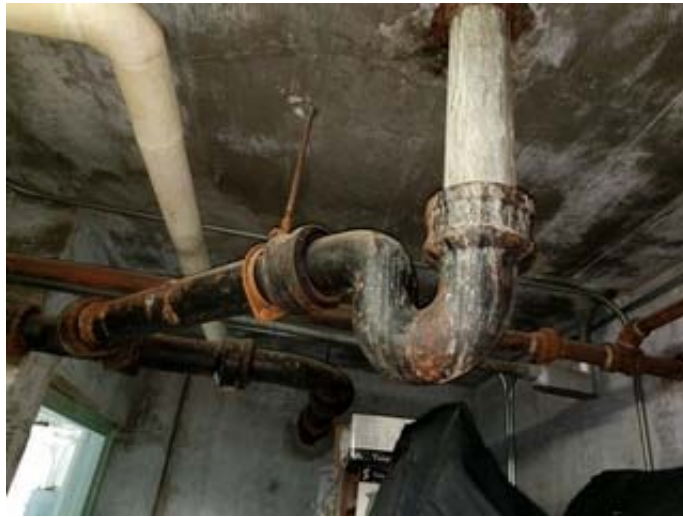
Cast Iron Sanitary Piping at Harman Elementary School
