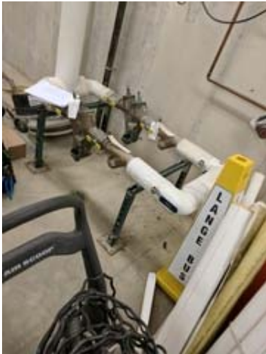
Dual 2" Backflow Preventers at Harman Elementary School
