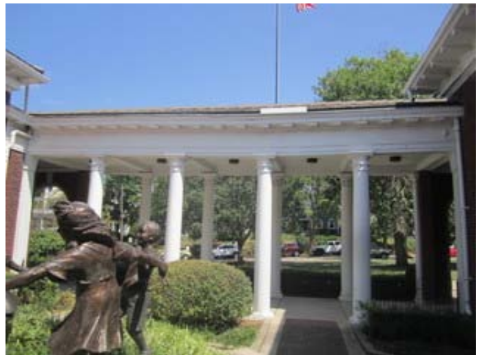
Portico With Sagging Roof Structure
