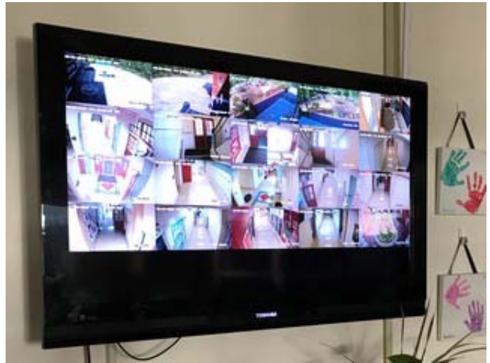
CCTV Type Security System Monitored In Administrative Area
