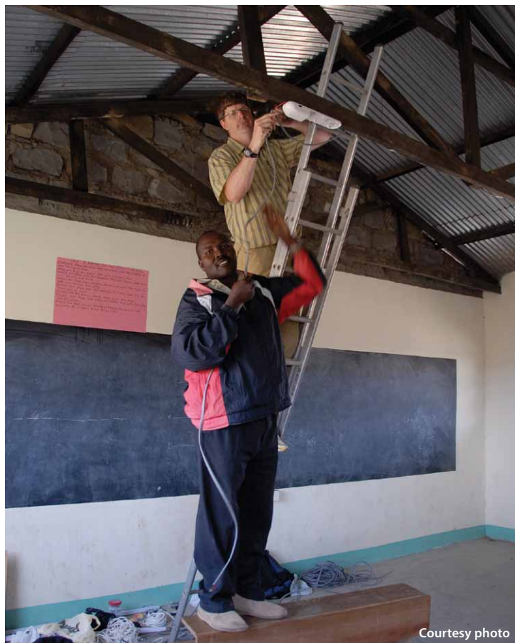
Kent Diamond and Moses Toroge work on the solar panel system at Lekanka Hills Primary School.
